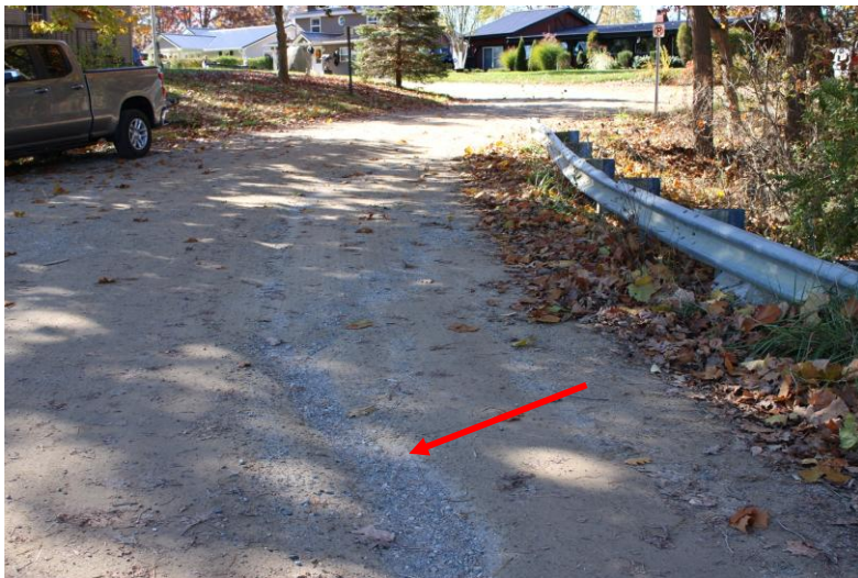
15. Gully erosion in road surface from previous runoff events.
