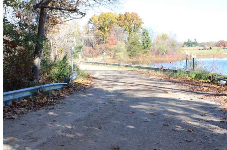
14. Road surface looking northward. Note erosion left of middle of road.
