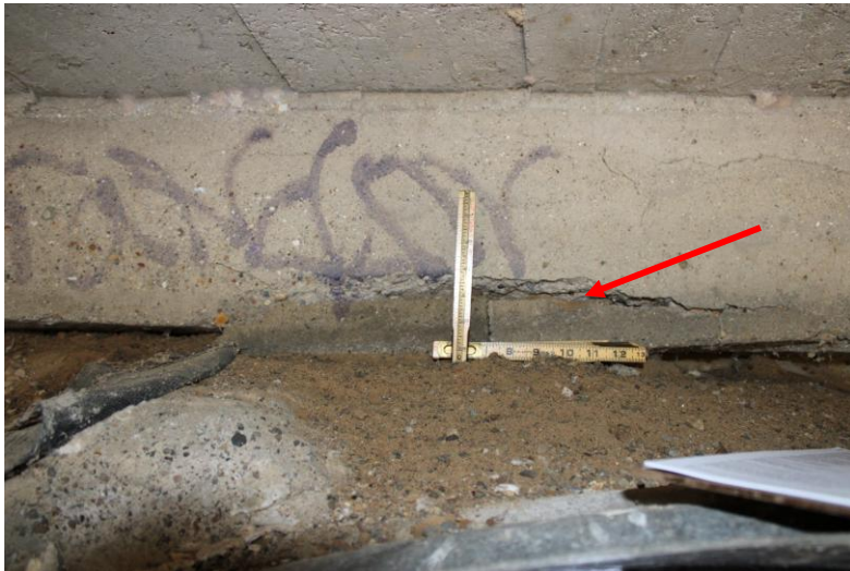
7. Crack in concrete on top of CMP
