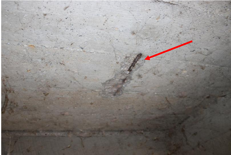
9. Exposed rerod in concrete box culvert about 3-ft inside of the structure
