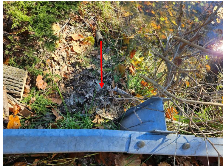
22. There were 2 small diameter CMPs here during the 2020 inspection, not visible now during this inspection. See 2020 report for picture comparison.
