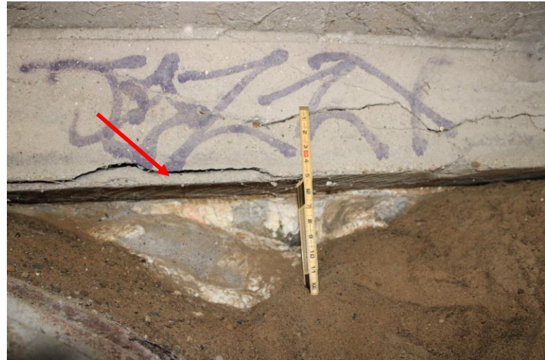
8. Crack in concrete towards right side of CMP. Compare with 2020 pictures
