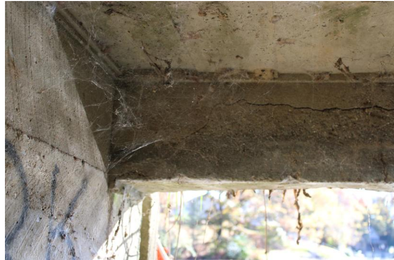
2. Spalling and cracked concrete along headwall of structure
