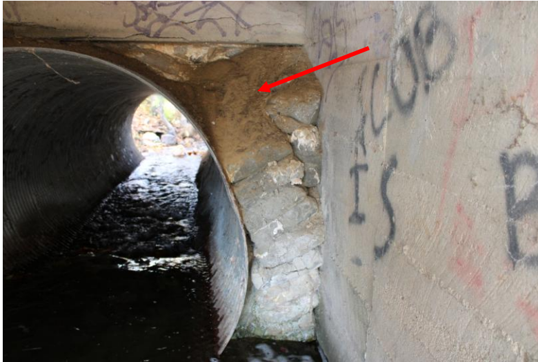
5. Right side of attachment note sediment spilling down headwall bags.
