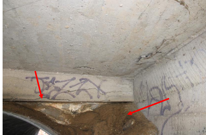
6. Cracking and sedimentation on right side of CMP
