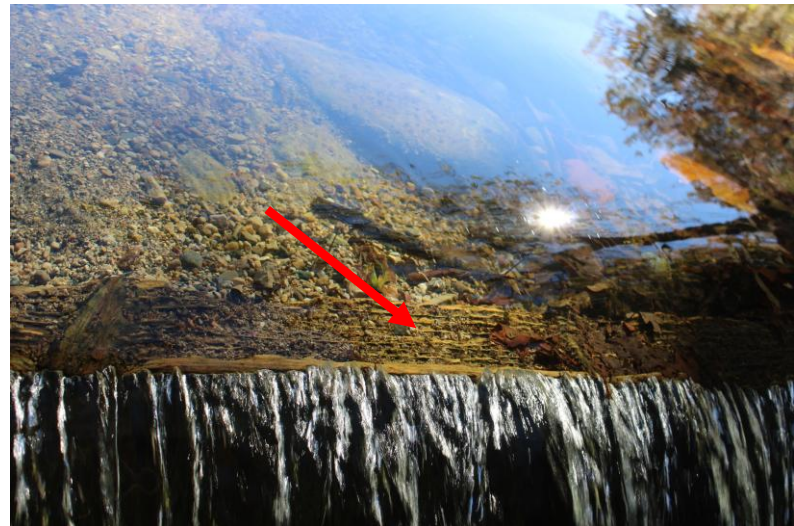
20. View of top weir stoplog showing the erosion of the wood grain.
