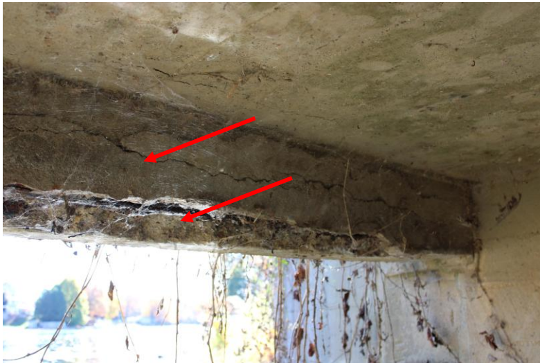
3. Spalling, cracked concrete and exposed re-rod along structure. When compared to pictures from the 2020 inspection, not much change.
